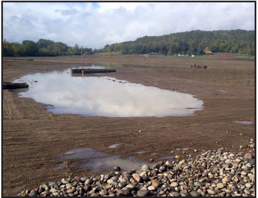
Vernal pool hydrology with jute fabric for erosion control and large wood to improve amphibian and reptile habitat (shown just after grading and prior to planting)
