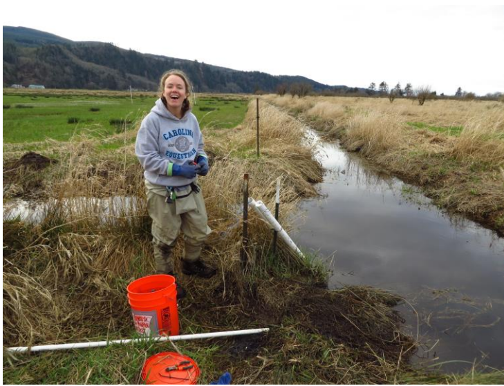
Figure B21. Laura Brown installing water level and conductivity/temperature dataloggers in the central ditch (Trib Upper sample station) at the SFC site. View is to the northwest.
