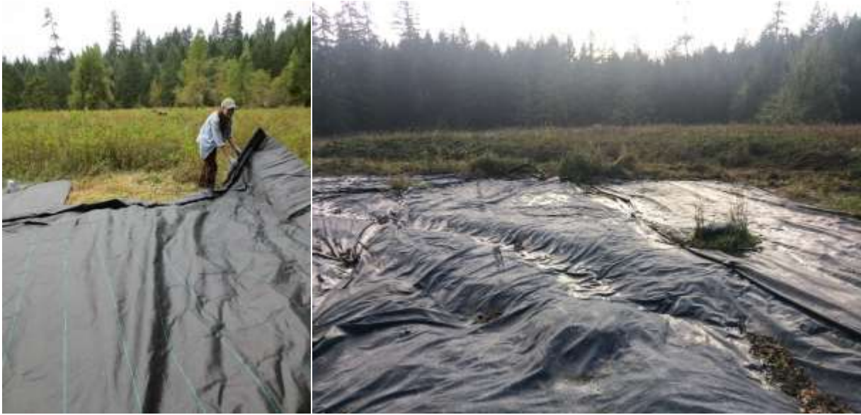
Figure 2. Shade cloth installation in 2014 (left) and condition in November, 2016 (right). (Photos: B. Axt and A. Neill)
