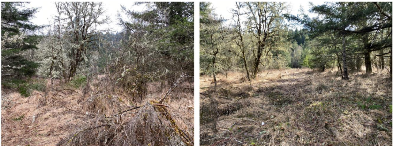
Figure 10. The southeastern corner of management unit E before (left) and after (right) cutting common hawthorn ( Crataegus monogyna ) and limbing Douglas-fir ( Pseudotsuga menziesii ) to establish a corridor between meadow patches. Photos taken in February 2023.
