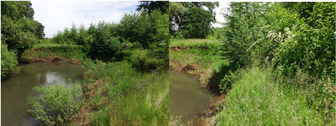
Figure 18. Photopoints RB1 (left) and RB2 (right) on Marys River, show erosion and undercutting of the banks. For precise location, see Appendix 2. Photo point locations at Herbert Farm and Natural Area.
