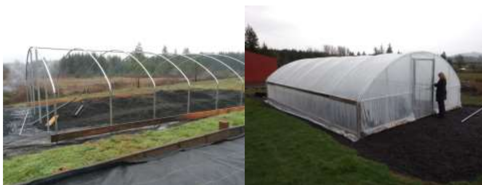
Figure 6. Left: Greenhouse being constructed at Natural Resources Department, December 2015); Right: Completed greenhouse in March 2016.
