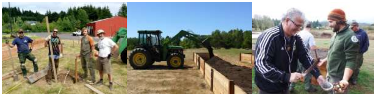
Figure 2. Left: Gabe Clift, Jeremy Ojua (Natural Resources Department), Guy Banner, and Peter Moore (IAE) building raised beds, July 2014; Middle: Filling the beds with soil; Right: Tribal Council member Jon George blessing camas bulbs held by Guy Banner, October 2014.
