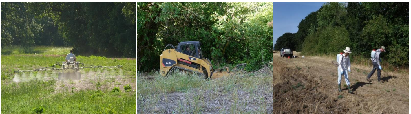
Figure 5. Left: Contractor from Habitat Restoration, LLC broadcasting herbicide in fallow grassland as part of site preparation before seeding native grasses and planting riparian trees and shrubs, June 2014. Middle: Skid steer mowing of riparian margin of blackberry, June 2015. Right: IAE staff spot spraying thistles, July 2016.
