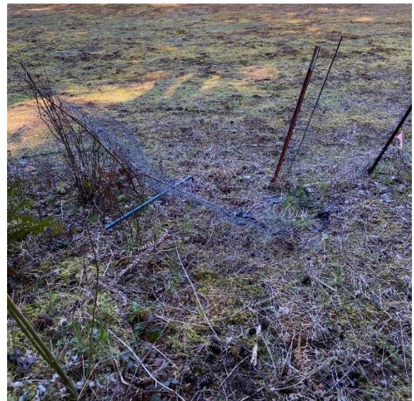
Figure 3. Wildlife enclosure with broken fence and bent and/or removed posts.
